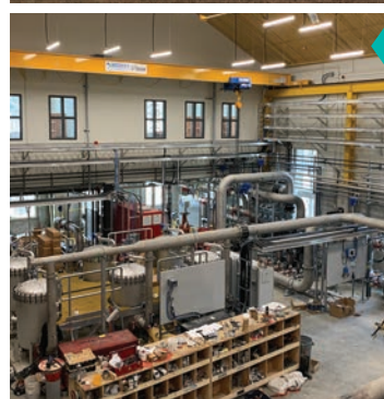
Associated Engineering received an Award of Excellence for the Dawson City Water Treatment Plant project in Yukon.
