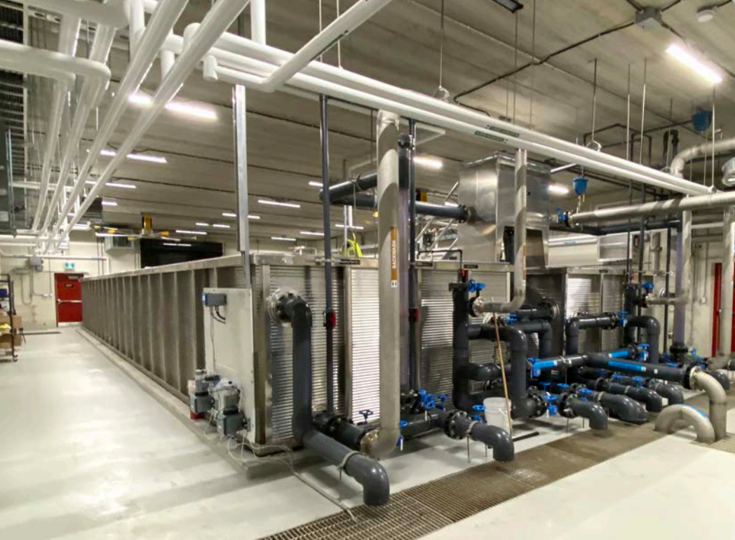
Neegan Burnside completed the engineering design, contract administration and inspection of a water treatment plant at the Kiashke Zaaging Anishinaabek–Gull Bay First Nation, located on the Ojibway nation on the shores of Lake Nipigon, approximately 200 km north of Thunder Bay, ON. Photo: Neegan Burnside
