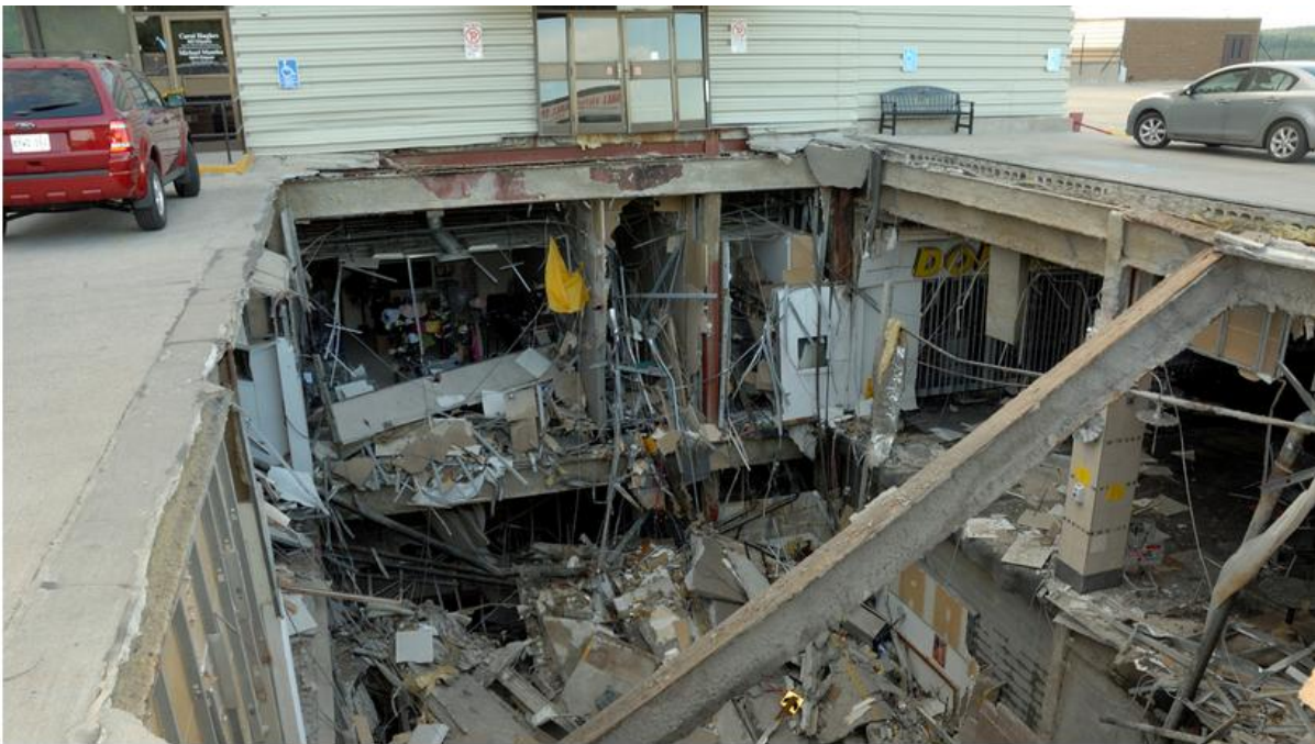
Ontario Provincial Police exhibit showing the collapsed parking lot at the Algo Centre Mall in Elliot Lake, Ont.
